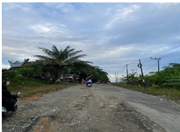
Figure 6. The damaged roads need to be repaired by the village government.
